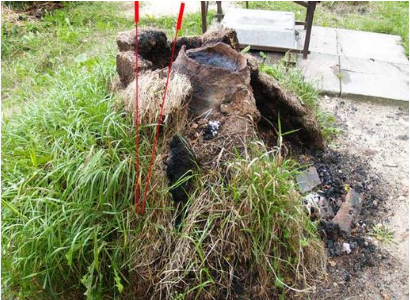
Side view, showing slumping of the furnace towards the extraction side (to right).
