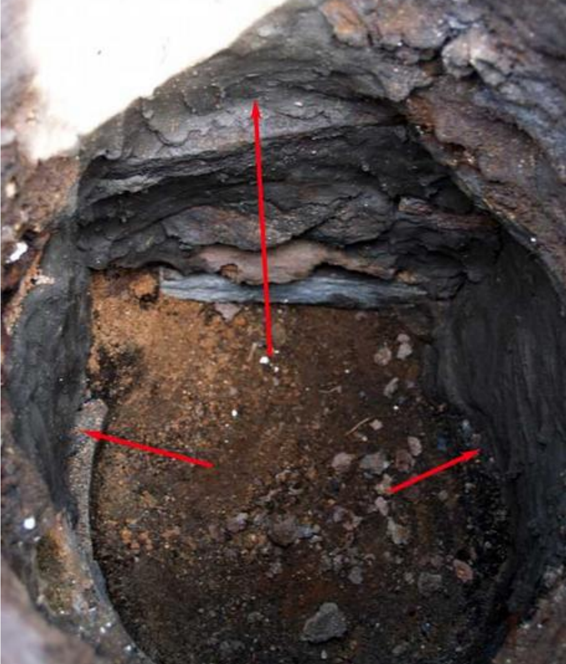
Interior after patching, larger areas indicated. At the top is seen the straight line of the lintel stone, which will support the tuyere tip when that is installed. The edges of the extraction arch stones are seen below the lintel.
